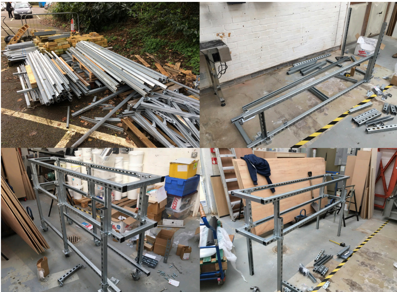
Fig 9: The construction of the extruder frame, starting from top left with the 'raw' material consisting of surplus Unistrut components, clockwise to the near completed frame in bottom left image. Photos: T. Jorgensen, 2020.
