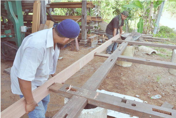
Figure 4: Modern Malay 'tukang' with his young apprentice installing the timber component in the assembly of a roof structure prior to construction on-site.
